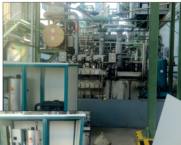
The CJC™ Varnish Removal Unit, VRU installed at Energyworks Valladolid, Iberdrola, Spain
