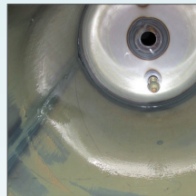
Clearly visible varnish at the metal surface BEFORE startup the VRU
