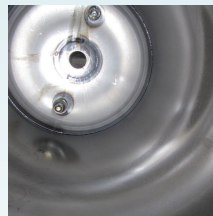
No more varnish at the metal surface AFTER startup the VRU
